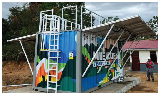
Mine Water Treatment Plant (MWTP)
